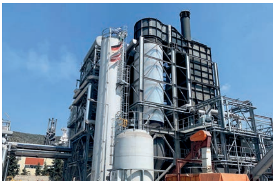
18.5 MW ORC BIOMASS PLANT | GREECE
