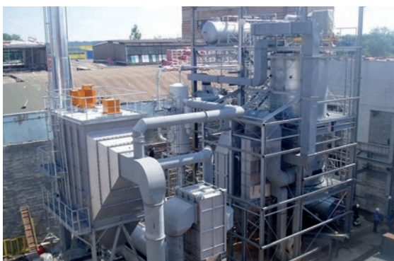
7 MW WOOD DUST 3-PASS HEATER | RUSSIA
